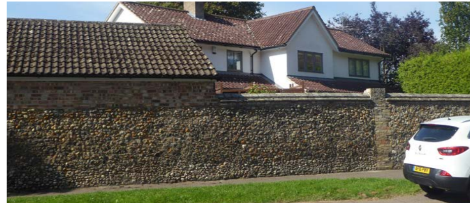
Fig. 54 - Traditional brick and flint walls - a distinctive feature of the village - used to define the edge of private spaces
