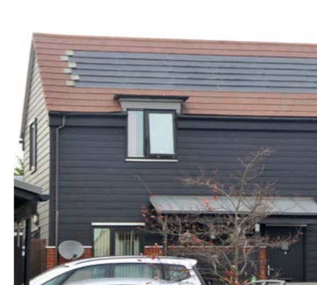
Fig. 55 - Solar panel design well integrated within the roof
