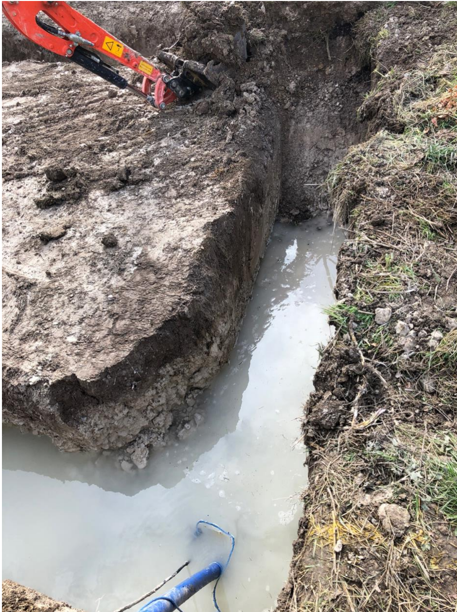
Figure A9. Ground water level at the rear of 60 Cow Lane 6-7 metres from southern boundary of the proposed development site, 4 April 2018. A pump was running at this point (blue piping) to drain the excavated trench. Ground water level was 40cm (0.4m) below the surface.
