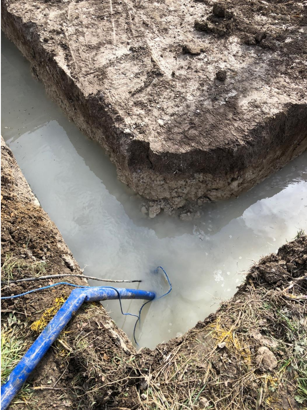
Figure A10. Ground water level at the rear of 60 Cow Lane, 6-7 metres from southern boundary of proposed development site, 4 April 2018. A pump had been running for 30 minutes to drain the excavated trench. Ground water level was 40cm (0.4m) below the surface.
