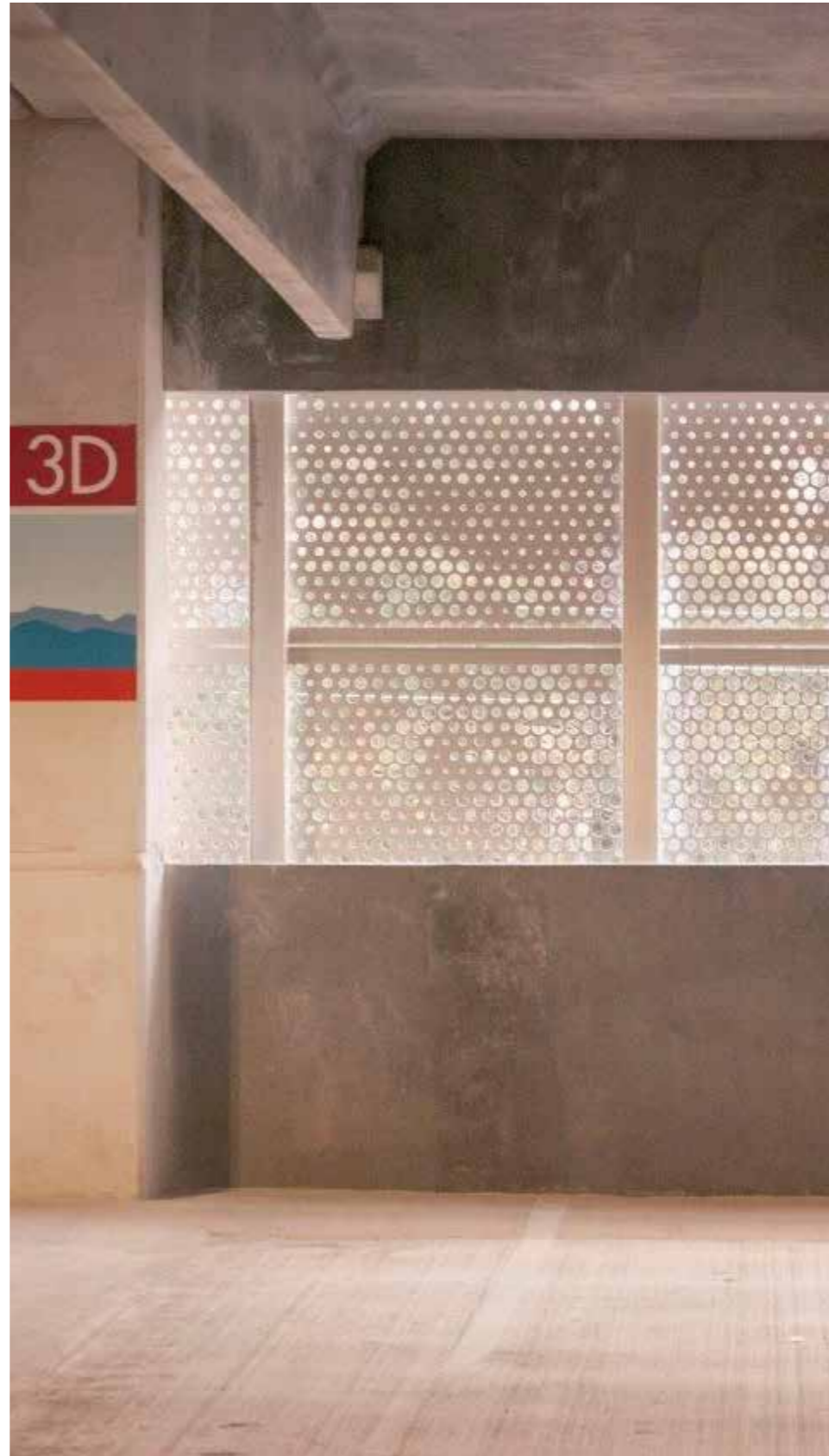
Raised RC crash barrier
